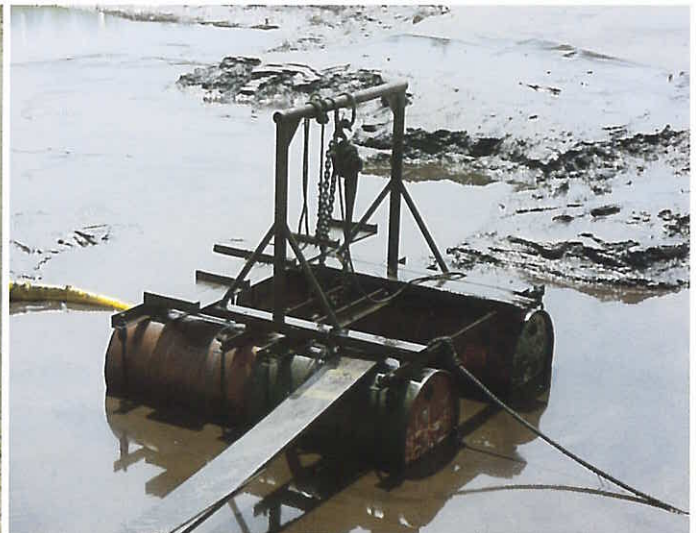
Close-up view of the pump float.
